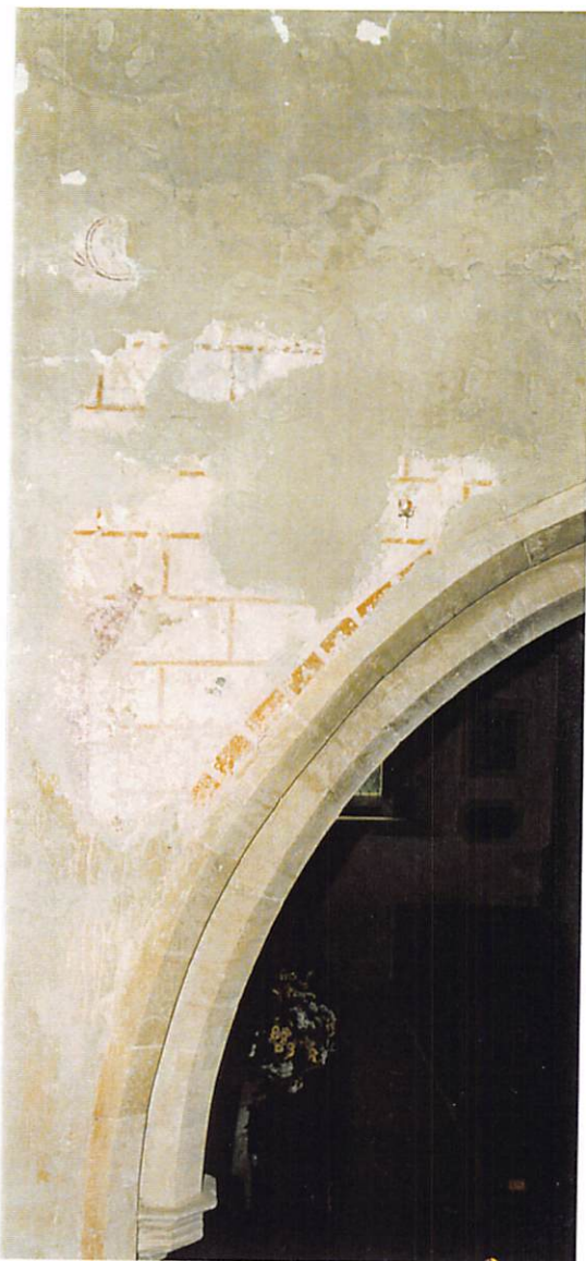
Plate 19. (Above) General view of the east side of the south wall. (Photo: Tobit Curteis Associates 1997)
